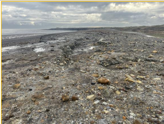
Recent overtopping damage to colliery spoil platform (3501/C01)
