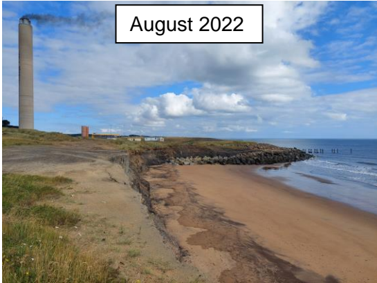
Eroding cliff to the north in August 2022. Tension cracks visible along the cliff top (3501/C01)
