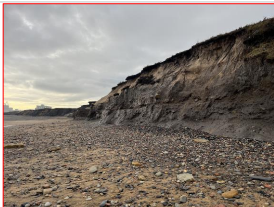
Accelerated erosion of the softer sand mantled on the colliery spoil platform (/3401C01)
