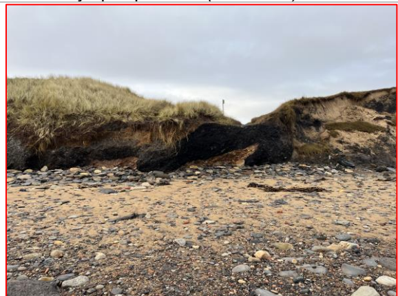
Beach access path, adjacent to Lyneburn Cottages travellers' site, inaccessible due to erosion (/3401C01)
