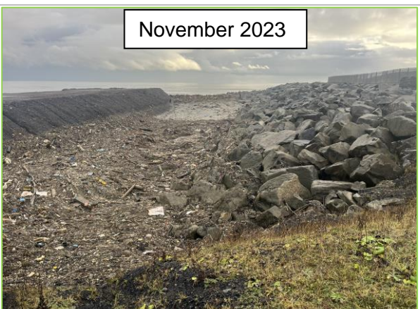
Significant volumes of storm deposits within outfall channel (/3401C07)
