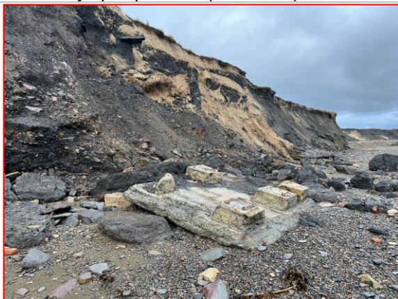
Concrete slab displaced due to recent erosion (/3401C01)
