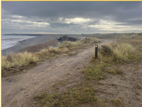
Eroding cliff to the north starting to impede the England Coast Path (3501/C01)
