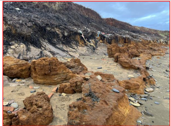
Erosion of the dunes previously protected by colliery spoil (/3401C01)
